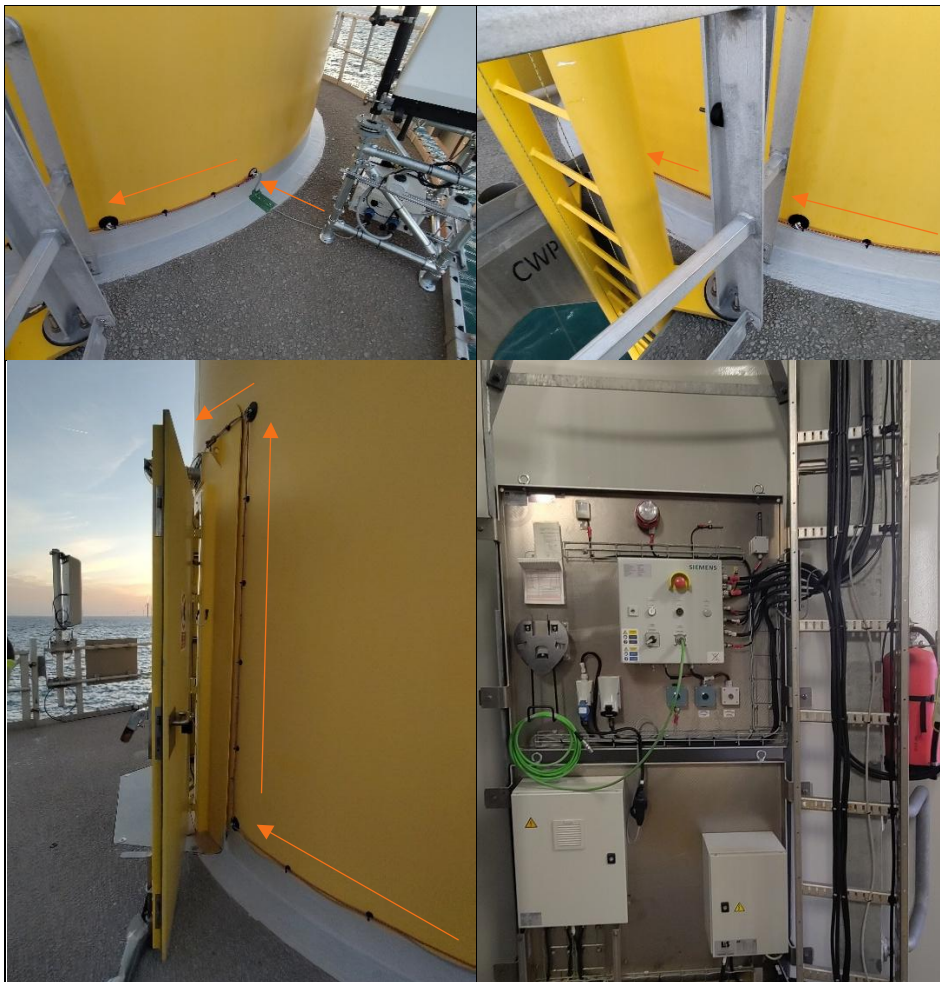
Figure 2-5: Cable routing indicated with orange arrows. Top left: 4G antennas on the lidar frame. Top right: power cable routed along the tower with magnets. Bottom left: power cable is routed along the tower entrance and entering the tower through the existing cable glands on top of the entrance. Bottom right: the power cable is connected to the 230 V service socket inside the tower base.
