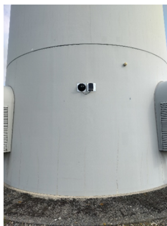
Figure 3.32: Picture of on tower microphone of Eologix-Ping in the Eemshaven
