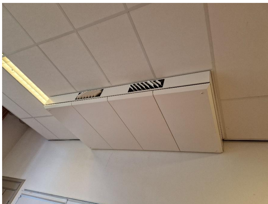
Figure 3-1 – Ventilation system after intervention
