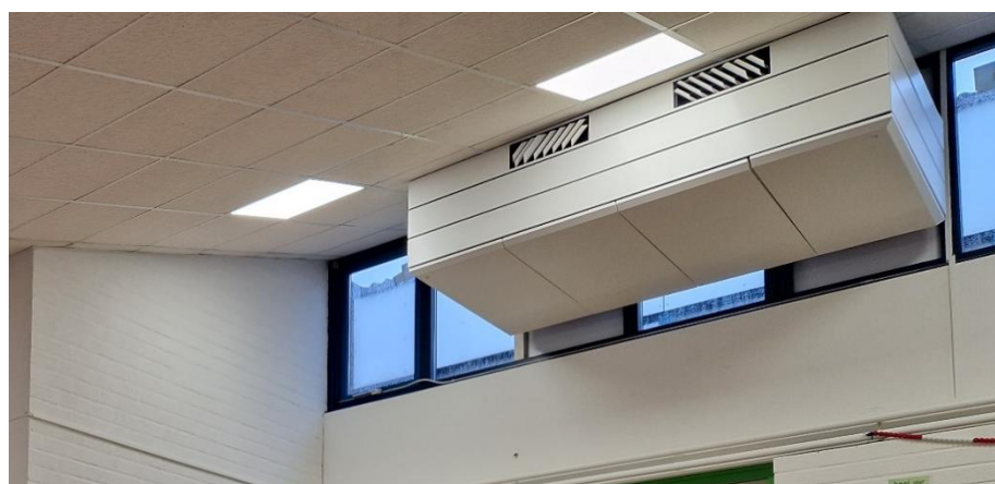
Figure 3-1 – Ventilation system after intervention
