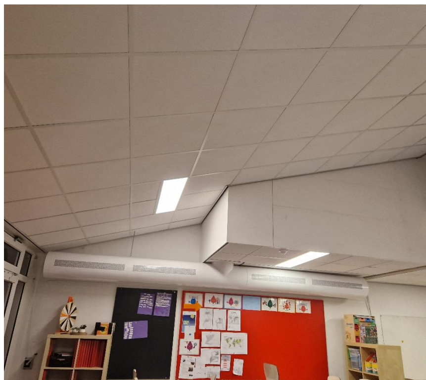
Figure 3-1 – Ventilation system after intervention C
