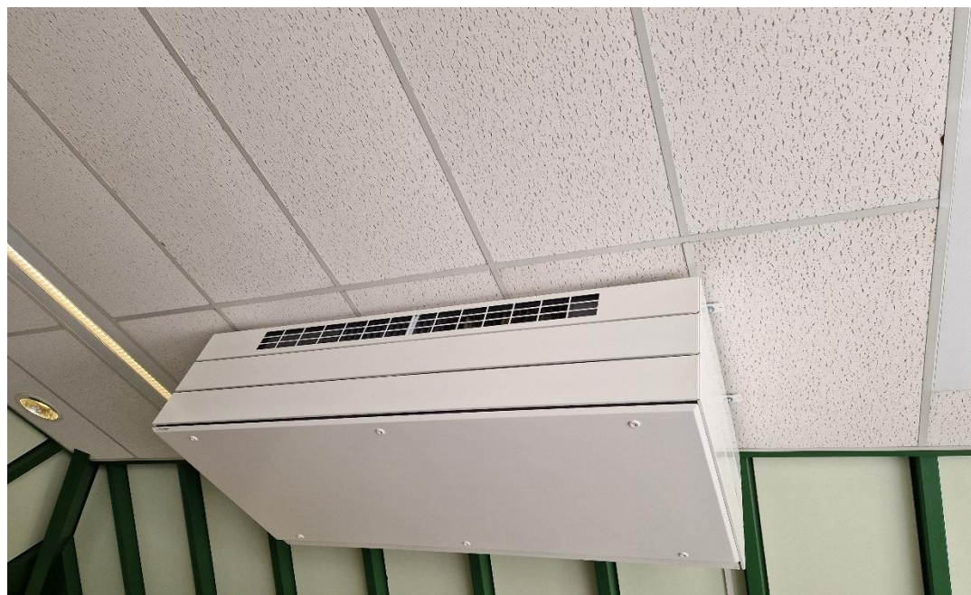
Figure 6-1 – Ventilation system after intervention
