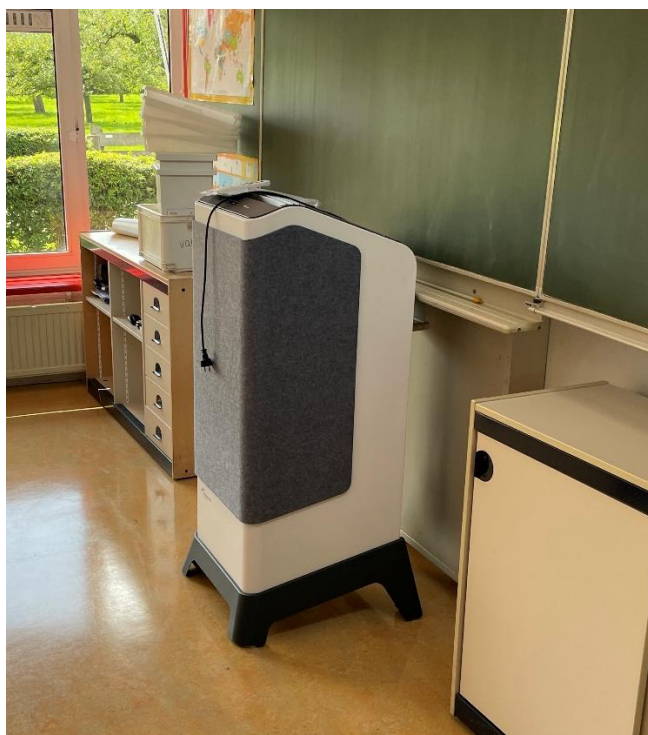
Figure 3-1 – Ventilation system after intervention
