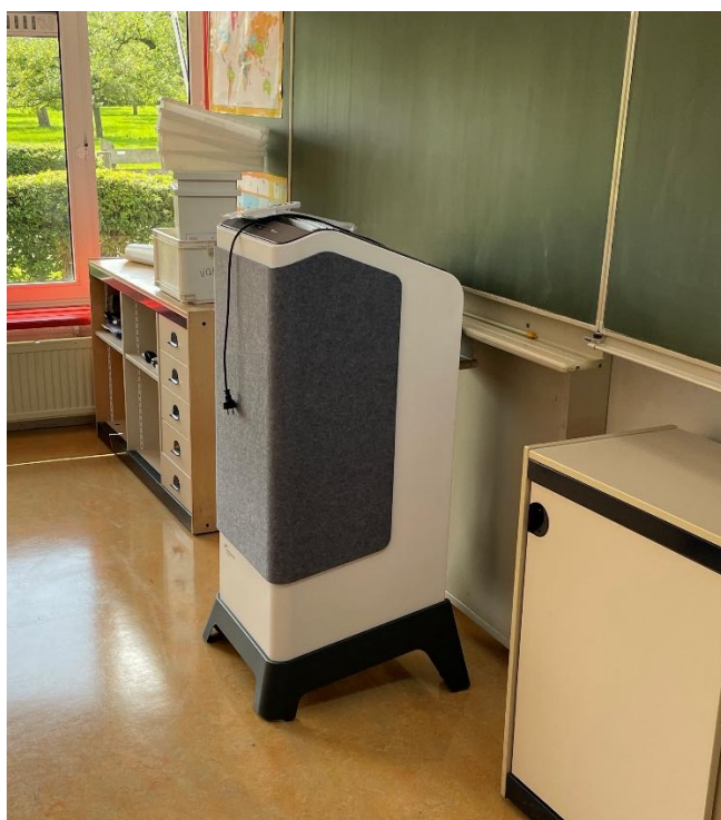
Figure 3-1 – Ventilation system after intervention
