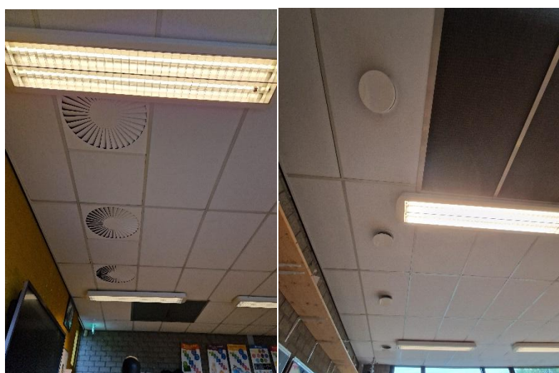
Figure 3-1 – Ventilation system after intervention
