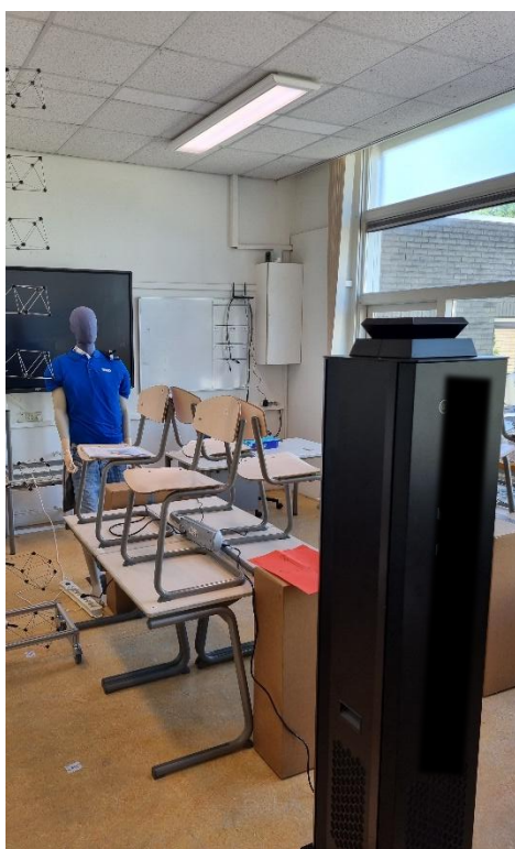
Figure 3-1 – Ventilation system after intervention A
