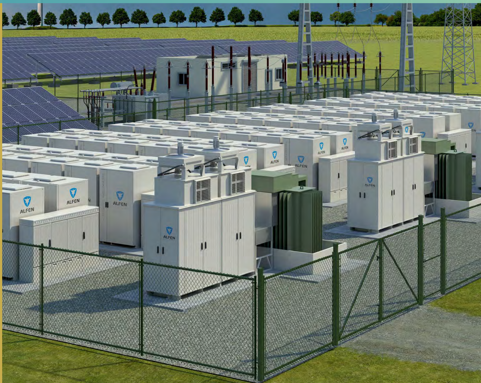
Netherlands FlevoBESS. Image credit: Alfen and FlevoBESS.
