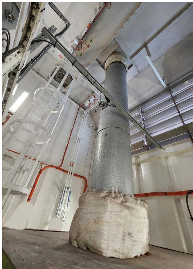
Figure 3.3: Position of Multronic NO x sensor just under the stack tower roof.
