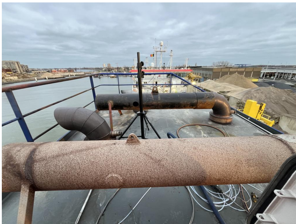
Figure 3.4: Straight pipe extension tubes with sampling hole on top of the stack.
