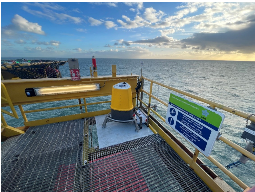
Figure 3.2: Lidar unit at L2-FA-1
