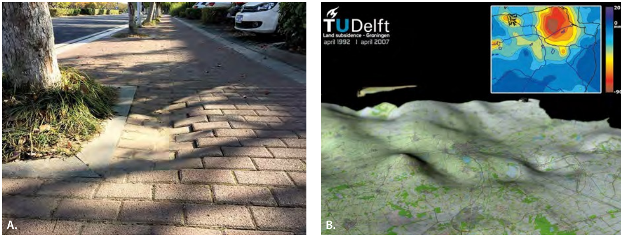
Figure 23.7. Subsidence occurs in many shapes and sizes. a) Subsidence bowl in a pavement. b) Subsidence bowls in the Groningen area, showing the cumulative subsidence between 1992 and 2007.
