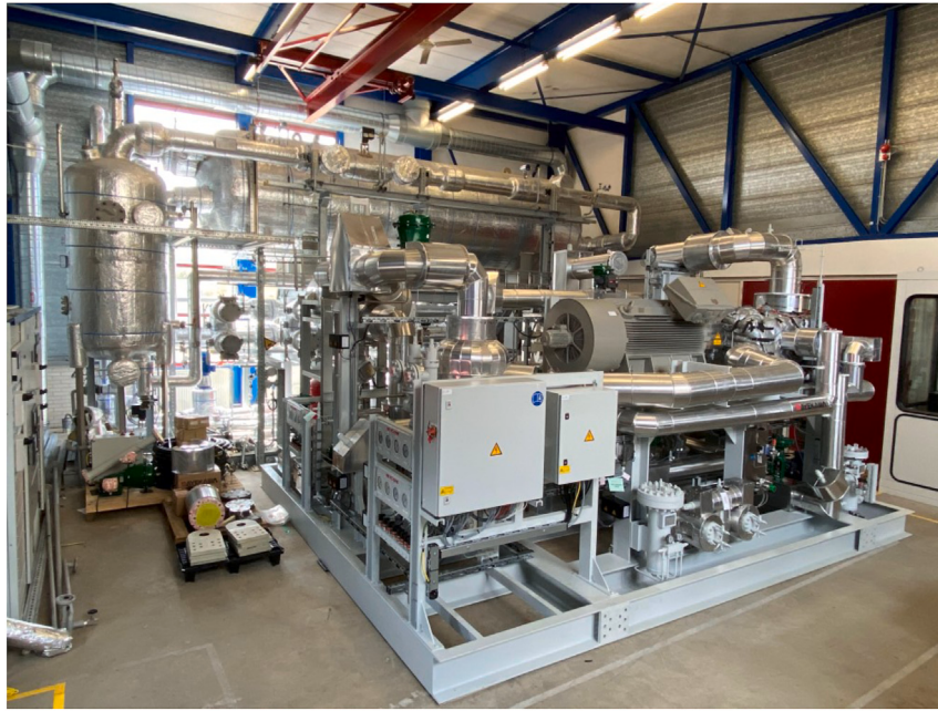
Fig. 2. TNO Carnot Laboratory including the pentane HP in the front and the test rig in the back.
