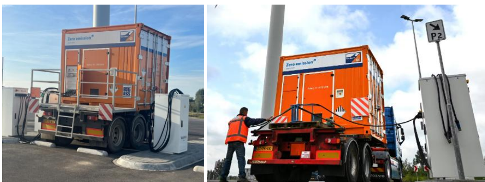
Figure 4.9. The container battery charging in the container charging area of WattHub. Connected to the AC charging (power lock) installation.
