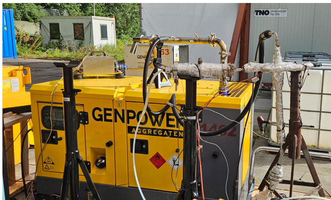
Figure 3.6: The diesel-powered 17.5 kVA genset.
