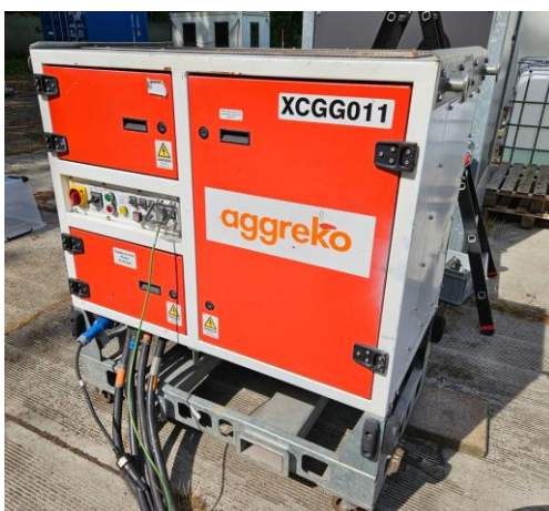
Figure 3.10: Load bank used to put load to the gensets and light pole.
