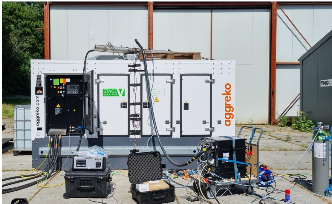
Figure 3.2: The diesel-powered genset at the test site.
