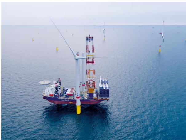
Figure 2.11: The AEOLUS jack-up vessel (JUV) from Van Oord installing a wind turbine (source Van Oord).
