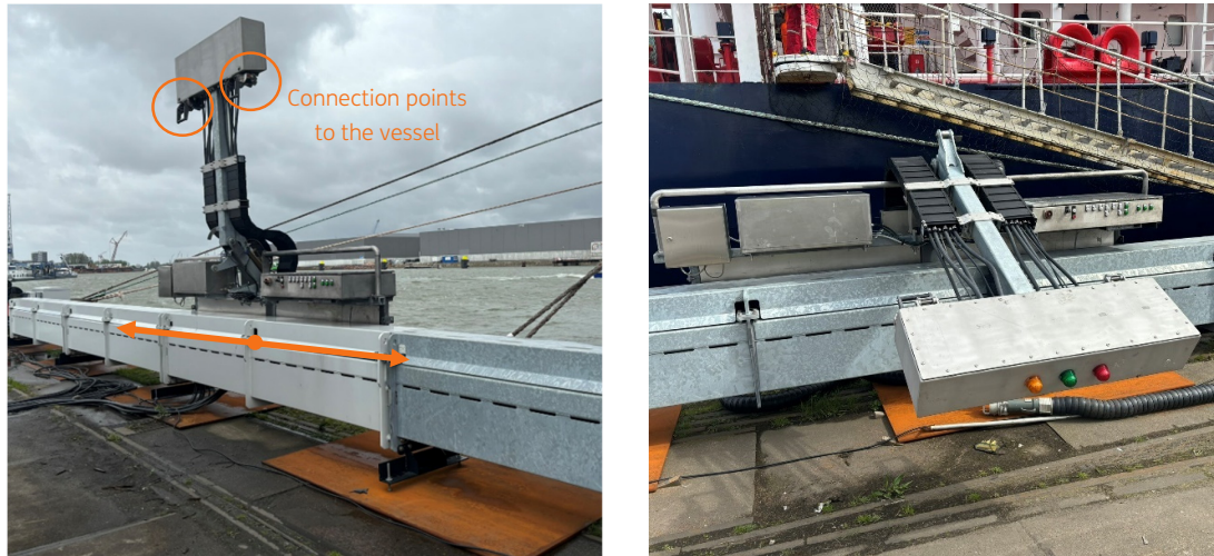
Figure 5: Photos of the IGUS Mobile Shore Power Outlet as installed in the pilot: Upward position (left), downward position (right).
