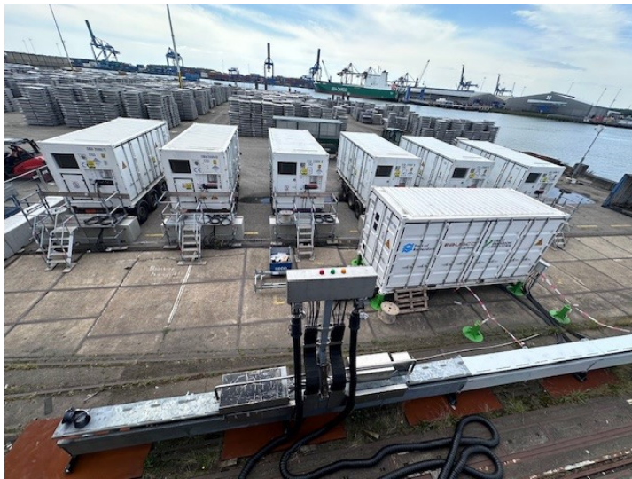
Figure 2: Photo of the shore power system on the shore side, taken from on board of one of the CargoW vessels.
