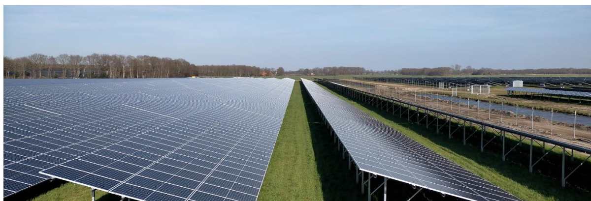
Figure 5: A view on a part of the Houtwal land-based solar park
