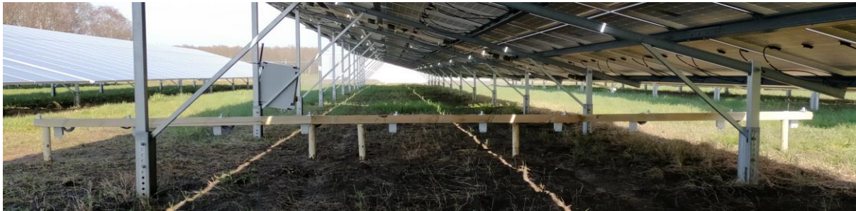
Figure 6: Light penetration sensors placed at the Houtwal land-based solar park.
