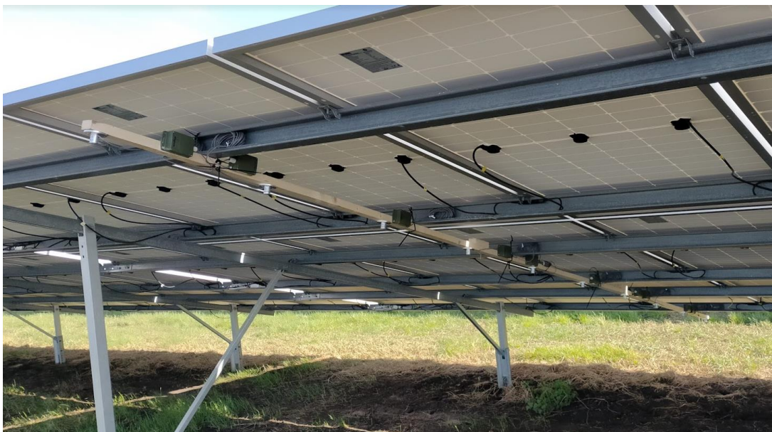
Figure 7: Rear side irradiation sensors at the Houtwal land-based solar park.
