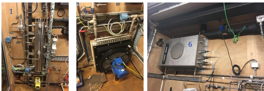
Figure 4: Pictures of main equipment for improved PEM testing station. The numbers correspond with the list above.
