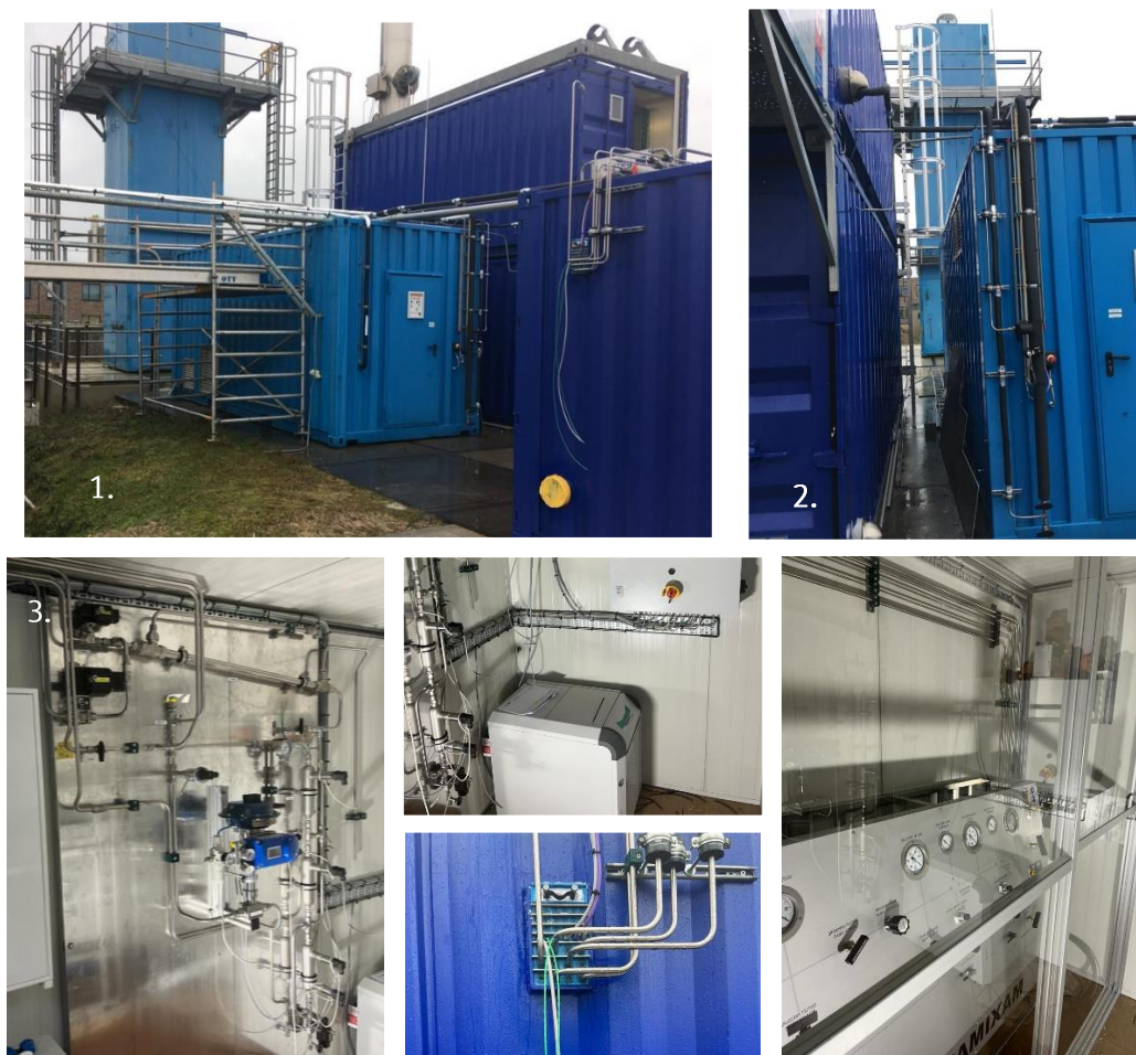
Figure 7: Pictures of the PEM-SEDMES connection. 1: Outside view showing connection between the nextgen container (light blue) and novel 10ft container with the hydrogen buffer. 2: Outside view with the connection between the SEDMES system and PEM. 3: Details inside and on the 10 ft container.
