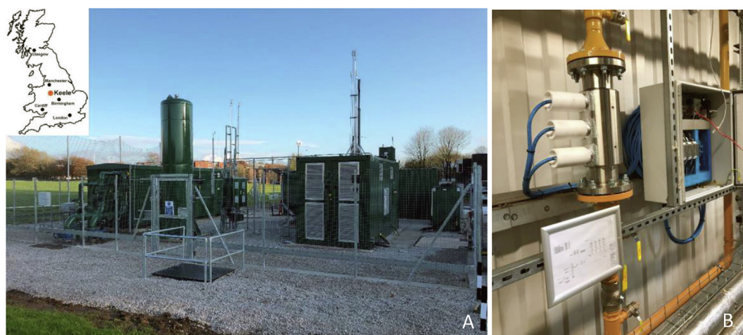
Fig. 3 – Keele university hydrogen production plant (A) and installed gas sensors in the supply line in a boiler house (B).
