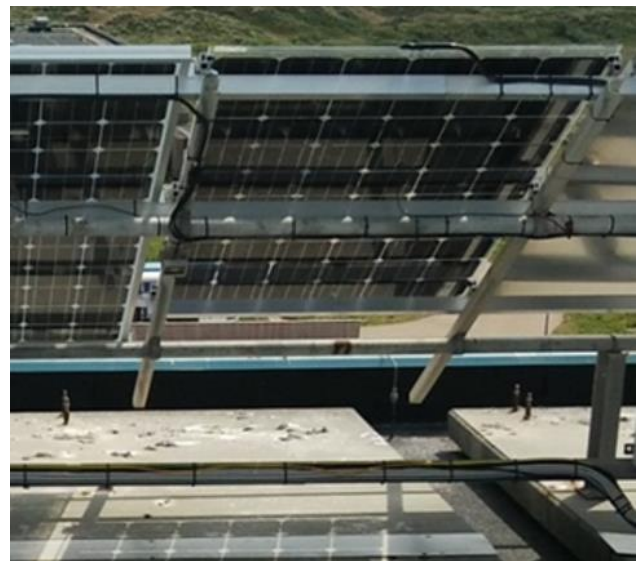
Figure 4 The patchwork of bright lines and hard shadow of the solar cells is visible in the bottom of the picture
