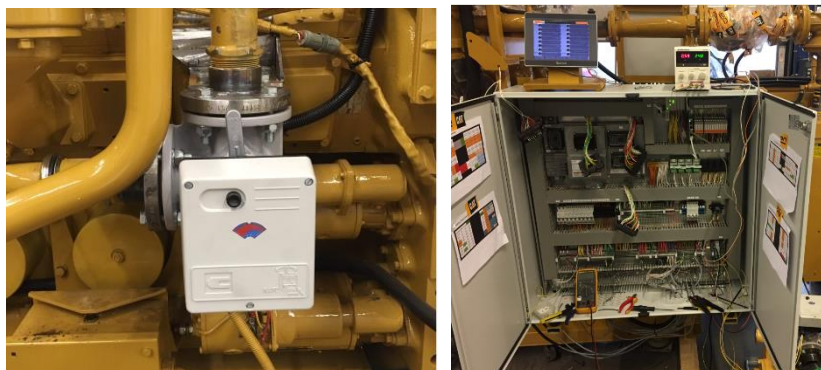
Figure 18: Cooling three-way valve with electric motor (a) and control system cabinet (b)
