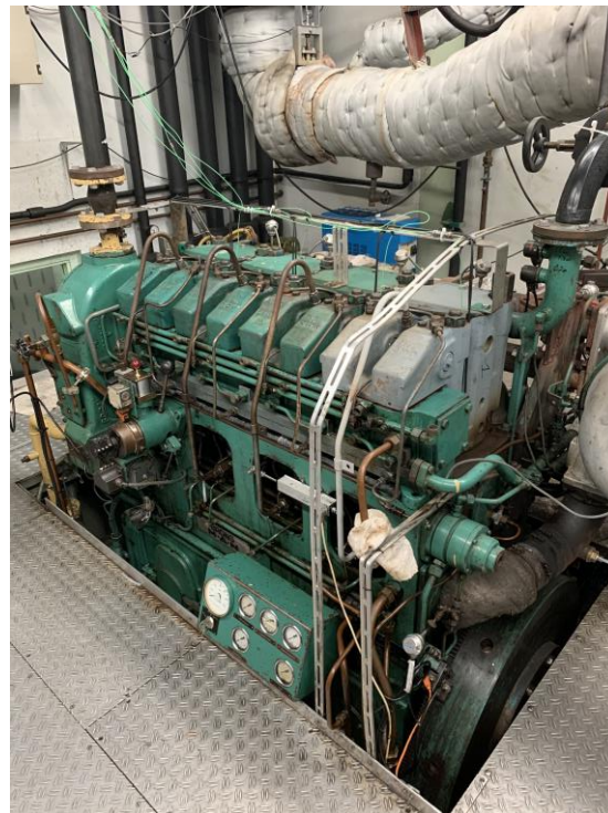
Figure 39: The diesel engine is a MAN 4L20/27 4-stroke Compression Ignited Diesel Engine
