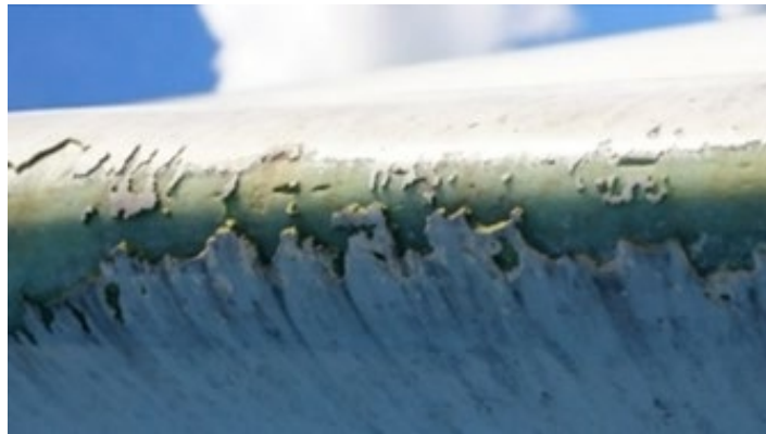
Figure 8 Leading edge erosion
