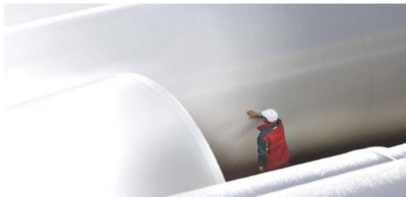
Offshore structures present some of the toughest corrosion protection challenges for coating systems. Hempel
