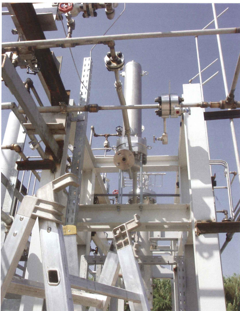
Hysep membrane module at the Tecnimont plant
