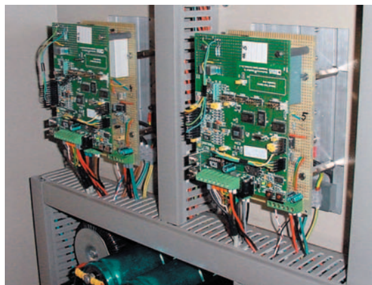
Unit for outdoor IV-measurements (left) and the control electronics (right).
