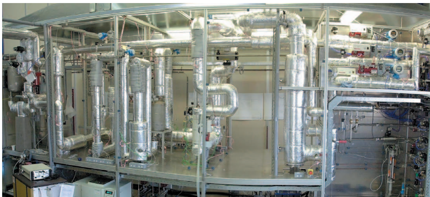
Panoramic view of the Fuel cell laboratory.
