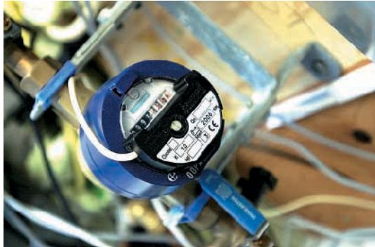
A water meter as part of the alarm system.
