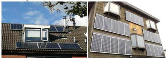
Figure 1: Typical PV systems as installed on rooftops and facades.
