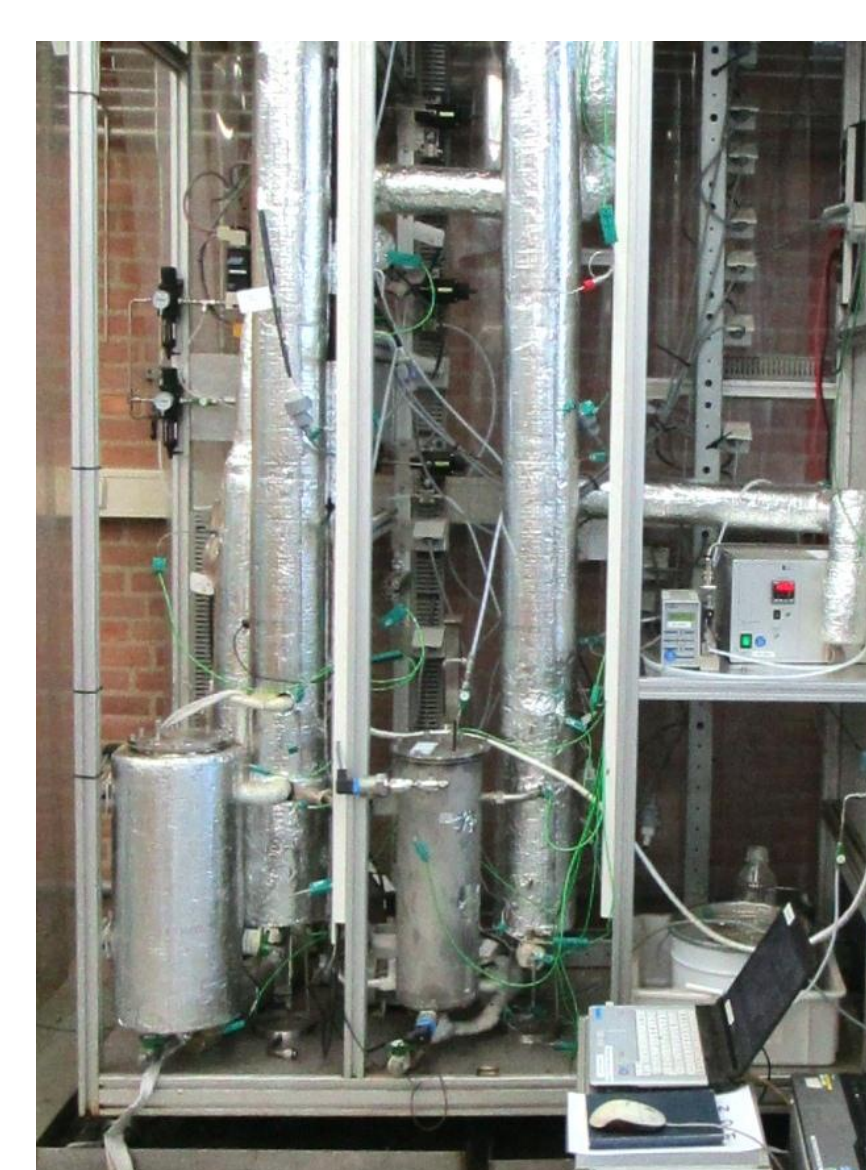
Bio-BTX scrubber unit (1 Nm 3 /h feed)
