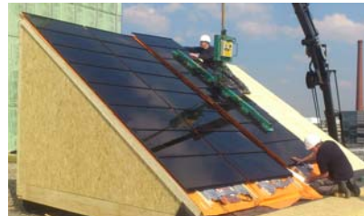
Figure 7 Crane mounting the prototype roof insulation integrated PV elements on the constructed artificial test roof in May 2014.
