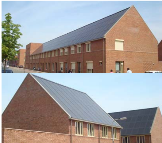
Figure 4. SCX Soloroof System as a BIPV full roof solution (Tilburg), 75 terraced dwellings
