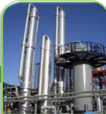
Gas cleaning OLGA
