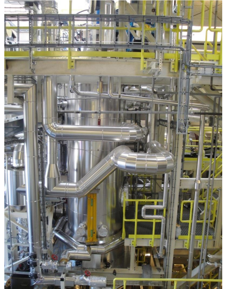
Torrefaction section of the demo plant
