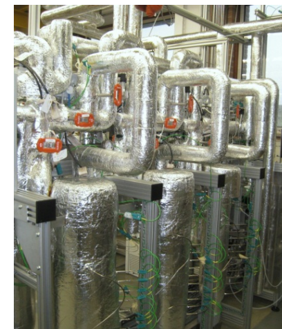
Methanation reactors 6 bar
