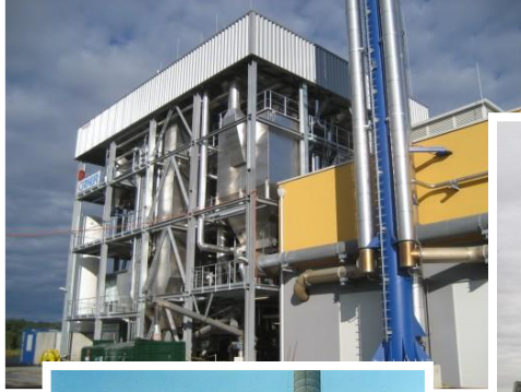
8 MW Oberwart, Austria
