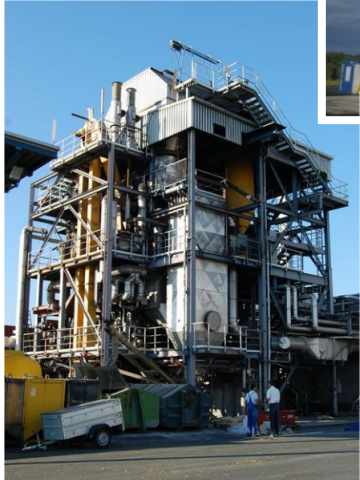
8 MW Güssing, Austria
