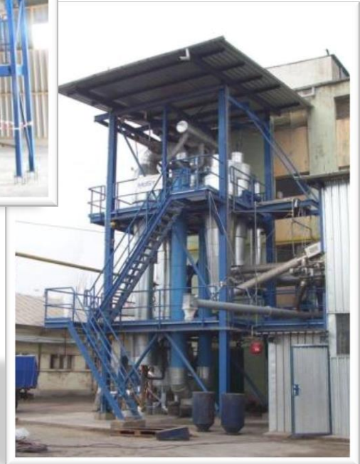
3-5 MW plant in Romania, sunflower husks, 2004
