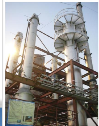
2 000 m 3 /h connected to MILENA
