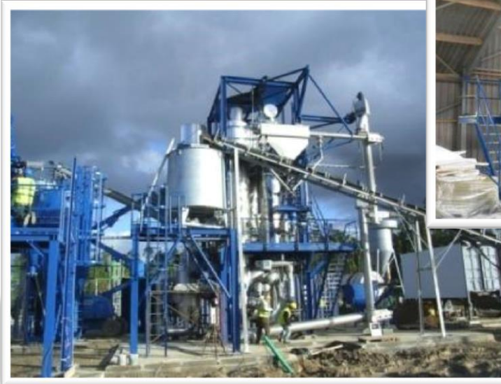
4 MW plant in Portugal, chicken manure, 2009
