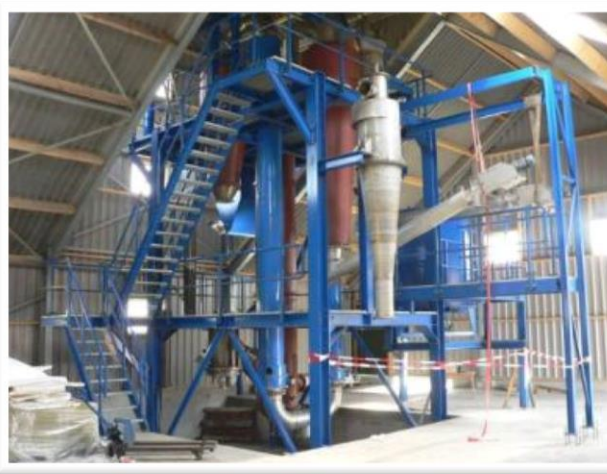
3 MW plant in Tzum (NL), chicken manure, 2006
