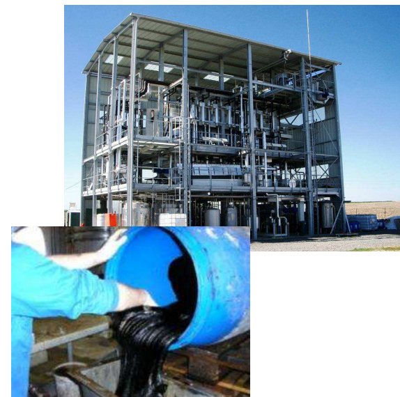
Acid organosolv Pilot plant ARD
