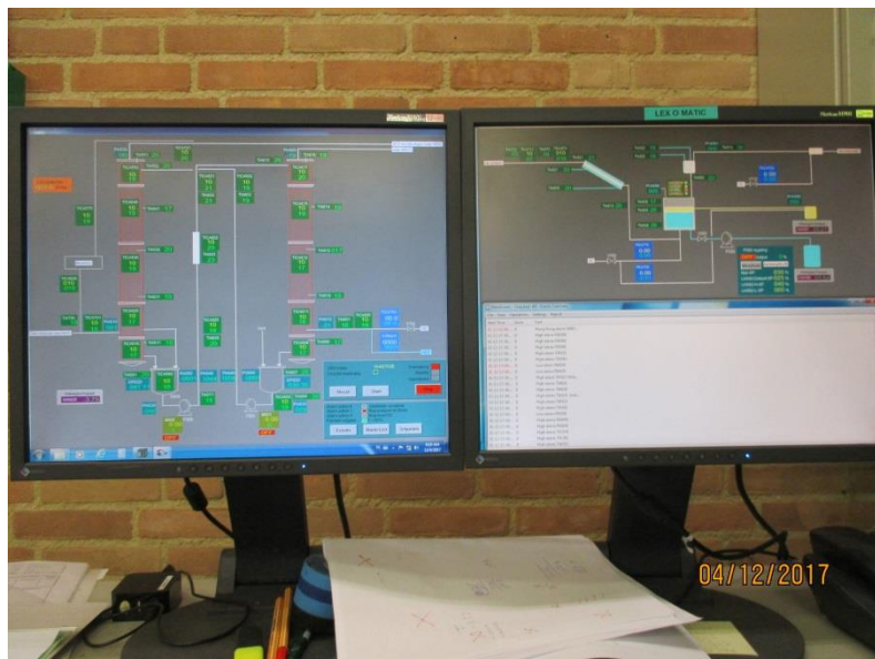
Figure 18. Computer controlled and automated system of bio-BTX scrubbing system.
