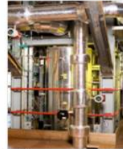
Torrefaction section of the reactor
