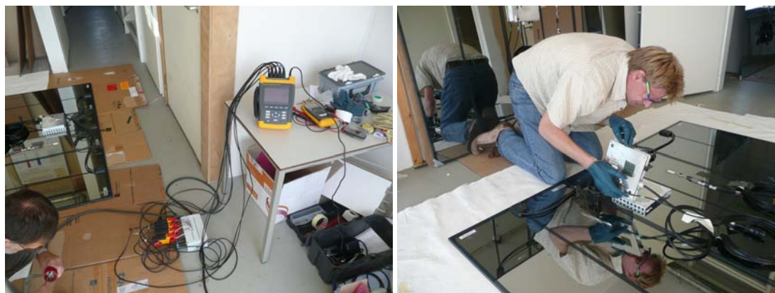
Figure 4.2 Measuring device and removing the failed inverter [ECN]
