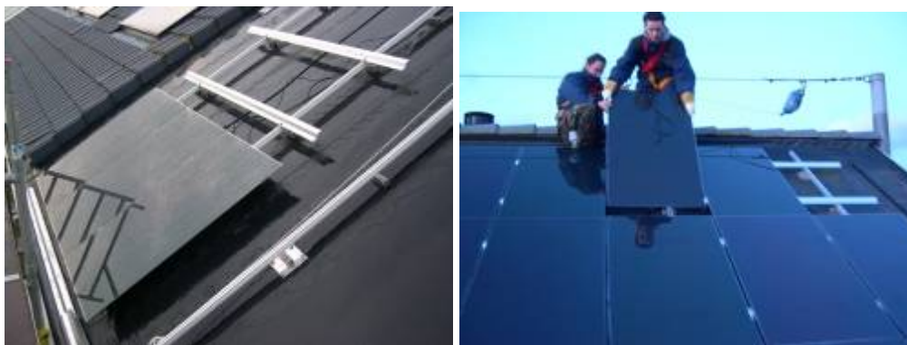
Figure 2.3 Integration of a-Si modules on the roof [ECN]
