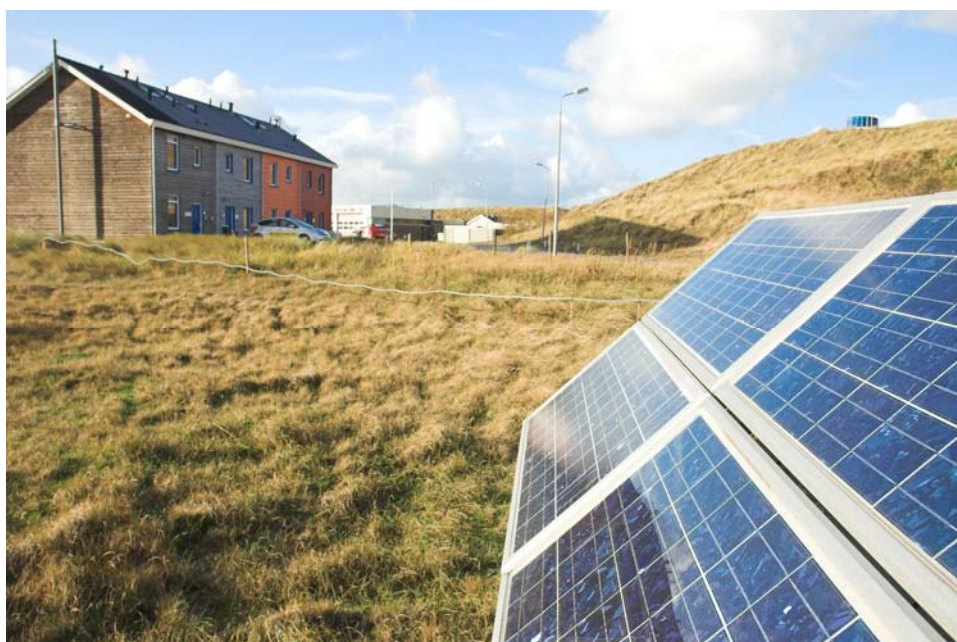
Figure 5.1 Photo of the solar panels connected to one of the test dwellings, in which the UPM resides
