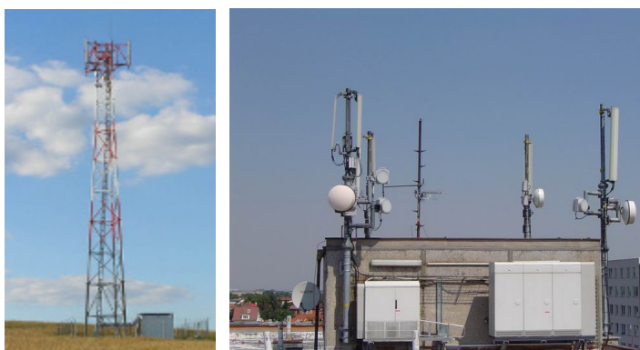
Figure 124: Mobile base transceiver stations and antenna system
