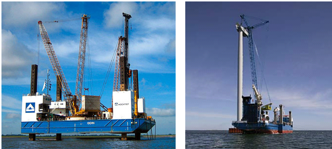
Figure 2.4: Examples of external cranes for replacement of large components; Jack-up barge ODIN (left) and crane ship Sea Energy (right)
