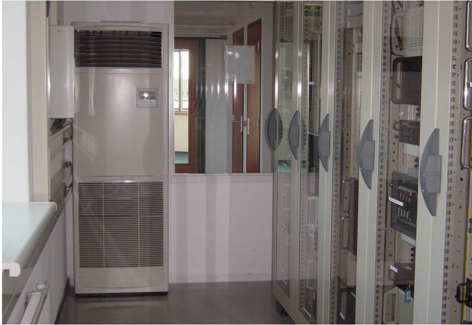
Figure 2.3 Server room in an office building. At the back on the left is an air treatment unit to provide cooling. On the right are the racks of computer equipment. Photo: ECN
