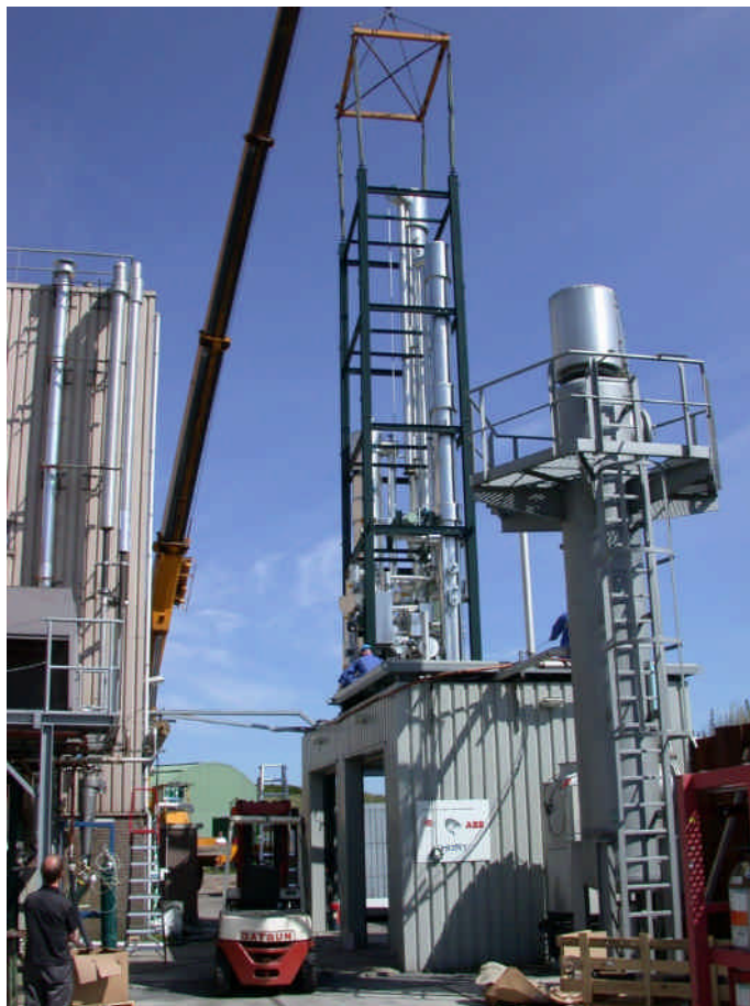
Figure 4.3. Positioning of OLGA skid in Dinkeldôme building. The ESP is visible on the foreground.
