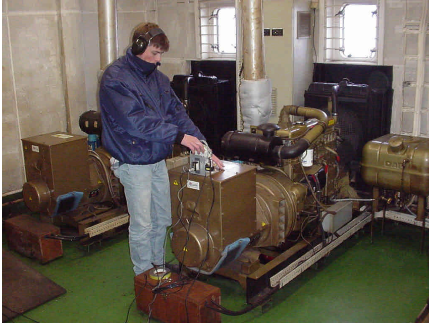
Figure 39. Vibration measurements at the generator.
