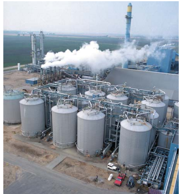
Ethanol pilot plant based on corn fibre and other cellulosic material, New Energy Company of Indiana, USA. (Courtesy DOE/NREL and W. Gretz)
