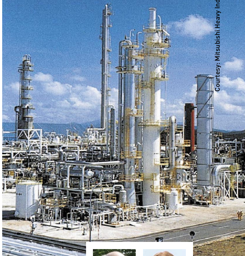
Figure 1: Capture installation at a small gas-fired power plant in Malaysia.
