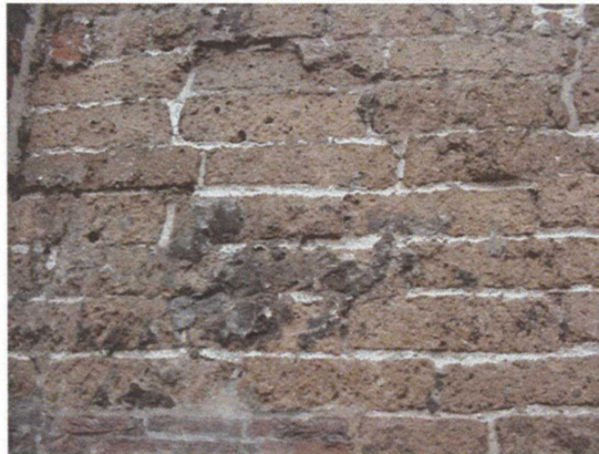
Fig. 3. Spalling of 11 th century Römer tuff on St. John's church, Utrecht (picture S. Brendle, 2002).
