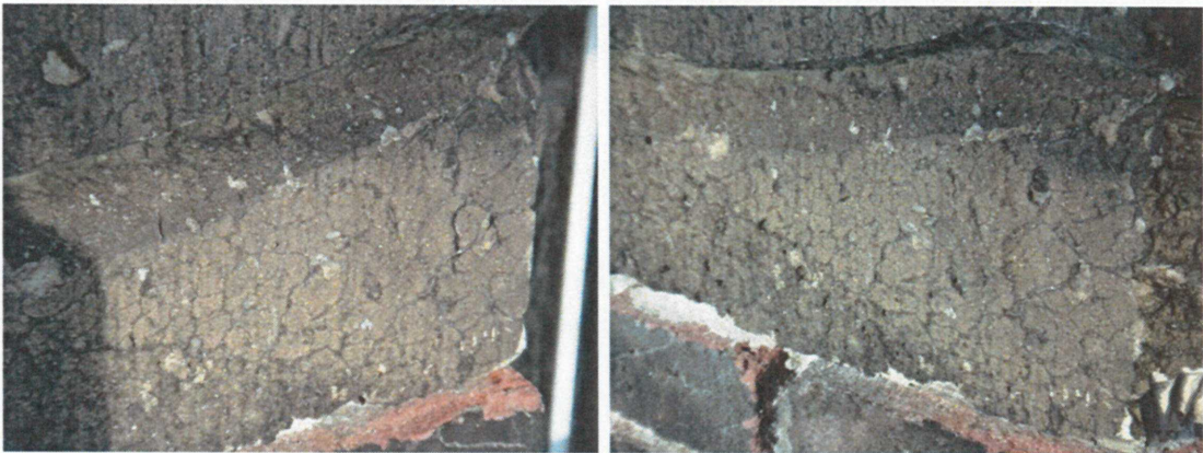
Fig. 8. Example of the formation of a hard, dark crust with craquelé on Ettringen tuff at the uppermost part of the tower of the Faculty of Architecture, TU Delft (pictures T.G. Nijland, 2014).
