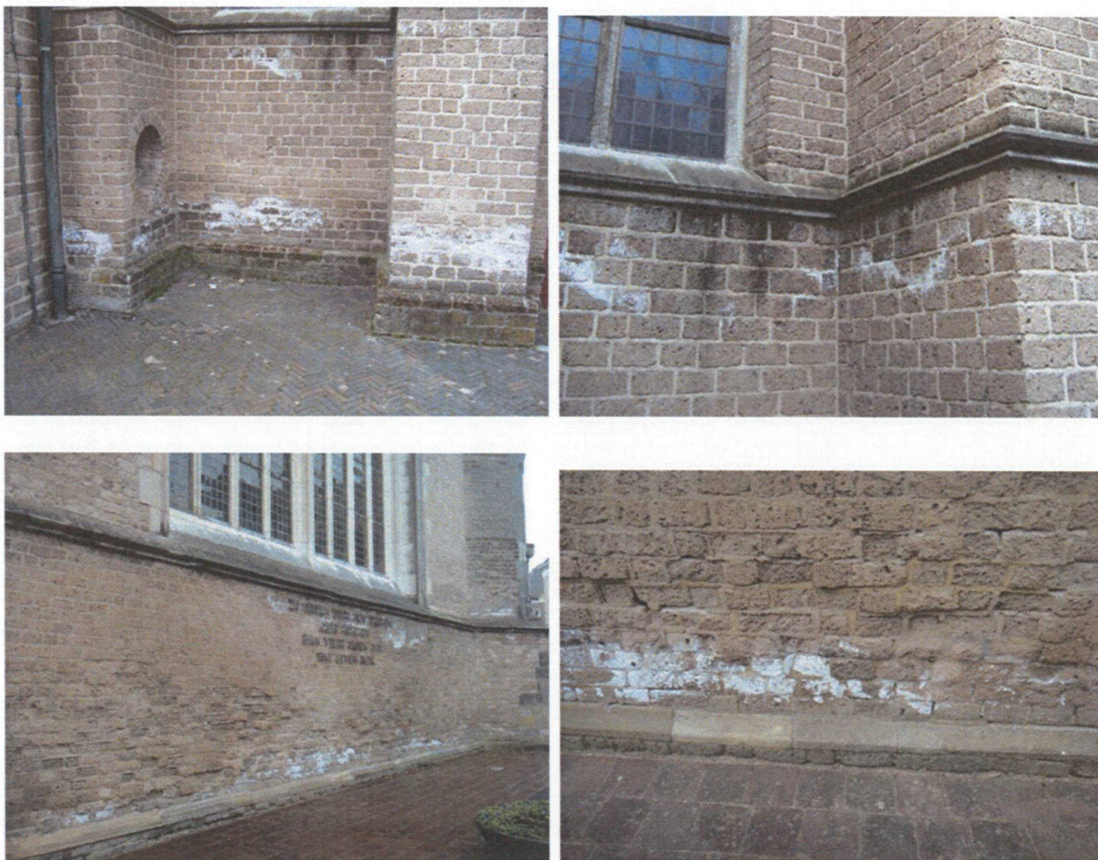
Fig. 11. Salt damage on Römer tuff due to \text{Na}_2\text{SO}_4 on St. Peter's church, Utrecht (pictures T.G. Nijland, 2010) and St. Lebuïns church, Deventer (pictures T.G. Nijland, 2013).
