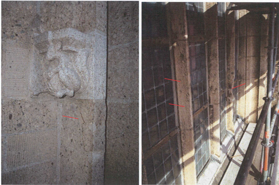
Fig. 5. Cracking in Ettringen (left) and Weibern (right) mullions at Eusebius' church, Arnhem and St. Peter's church, Leiden, respectively (pictures T.G. 2009 & 2005).
