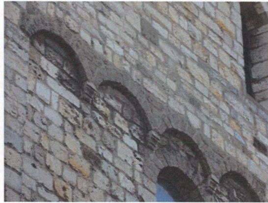
Fig. 5. Römer tuff tracery in Kunrade limestone masonry at the old Romanesque basilica St. Plechelmus, Otger & Wiro in St. Odiliënberg (picture T.G. Nijland, 2016).
