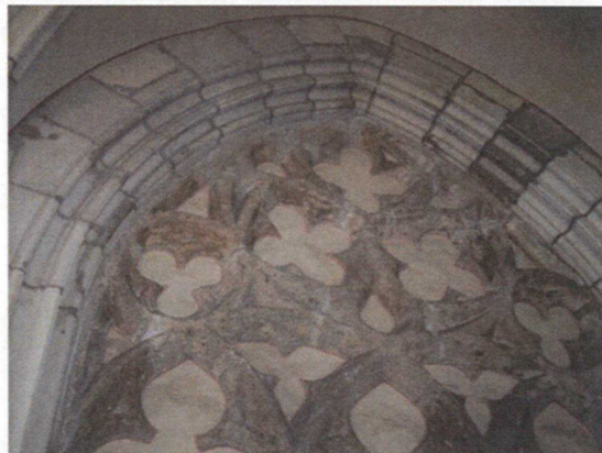
Fig. 9. 15 th Century blind tracery in the cloister of the Utrecht Dom cathedral (picture T.G. Nijland, 2005).
