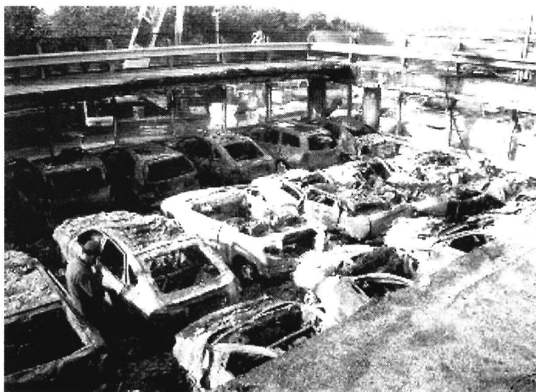
Figure 1 Picture after the fire in the car park near Schiphol airport (picture from [1])
