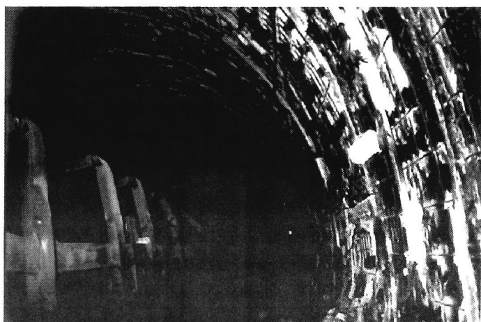
Figure 1: Fire damage in Channel tunnel
