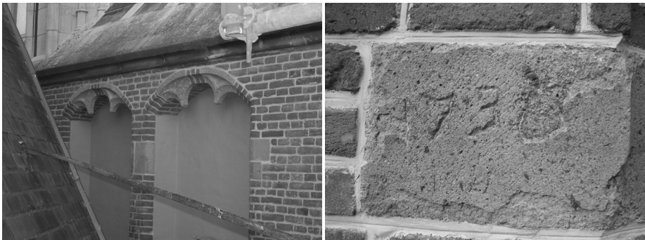
Figure 9. Blocks of Laacher tuff on the crossing tower of St. John's cathedral, 's-Hertogenbosch, dating back to the 1730's.
