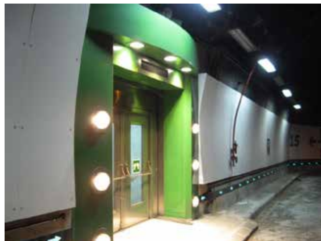
Illustration 14b - Cadi tunnel (flashing exit location indicators combined with flashing exit route indicators)
