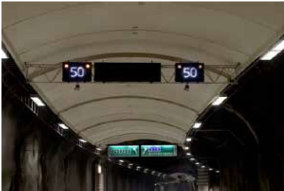
Illustration 6a - Southern link tunnel Stockholm (Sweden)
