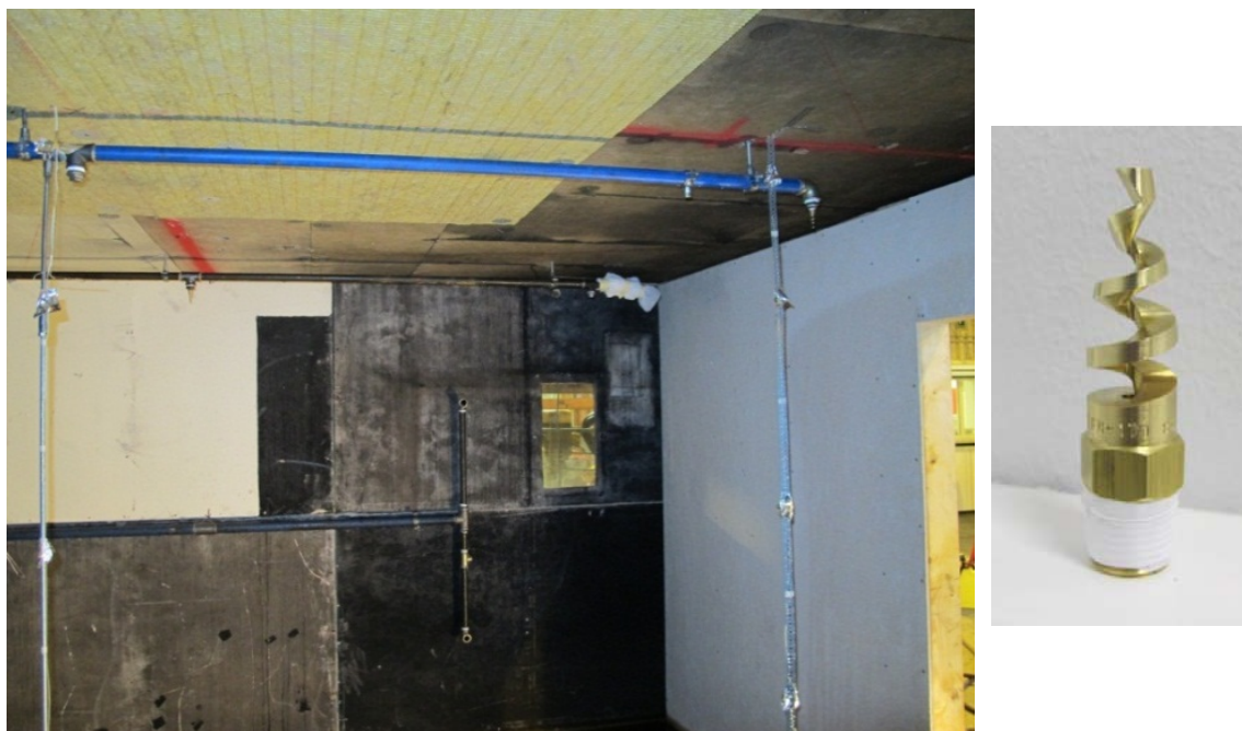
Figure 5 Low pressure water mist system. Parts of two of the longitudinal pipes and four nozzles are shown. Close-up of the BETE TF8-170 nozzle is shown on the right.
