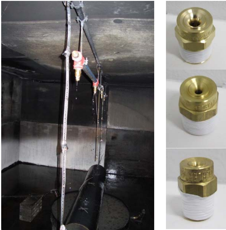
Figure 6 Drencher system and LECHLER nozzles 460.928, 460.728 and 460.608 from top to bottom.
